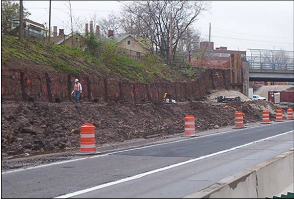
Whole face of initial stage of excavation readied with anchors, attachments and steel reinforcing with drains, for concrete application.
