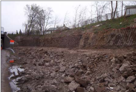
Bank is excavated in first lift ready for first row of anchors.
