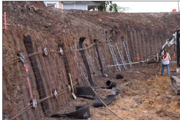
Placement of screw anchors and details on face reinforcing and anchor plates with tension nuts on thread-bar.
