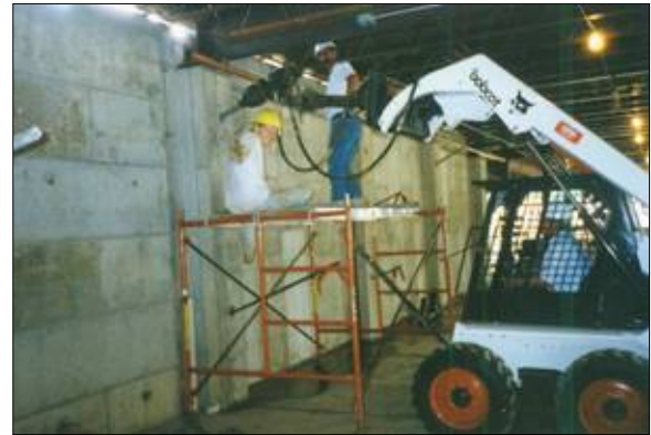
Installation of screw anchors through failing foundation wall to ensure long term stability easily and quickly.
