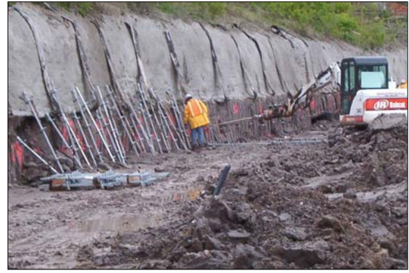
Second stage of excavation and anchoring continuing. First stage is completed and holding above the deeper excavation and ongoing anchor installation.
