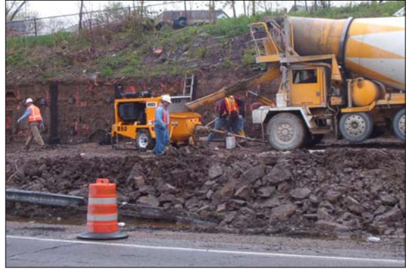
Shot Crete pump and concrete supply truck used during typical concrete applications to tieback walls.
