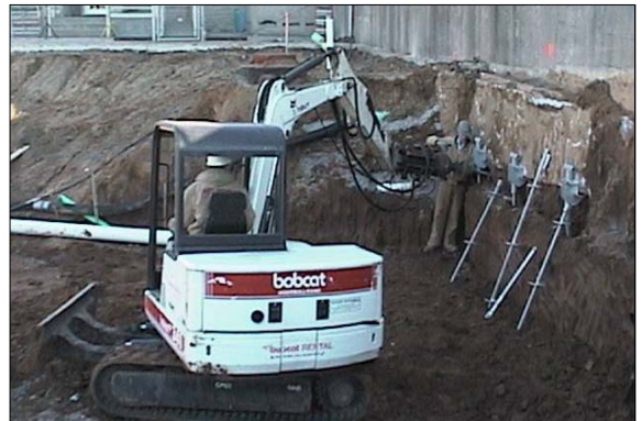
Installation of tieback anchors alongside helical pilings capped with galvanized steel underpinning brackets used to temporarily underpin the footings of the overpass alongside the excavations for the new roadway.
