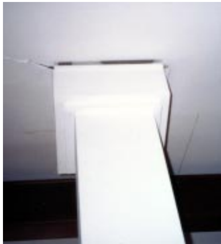
1"+ gap can be seen between column and ceiling.
