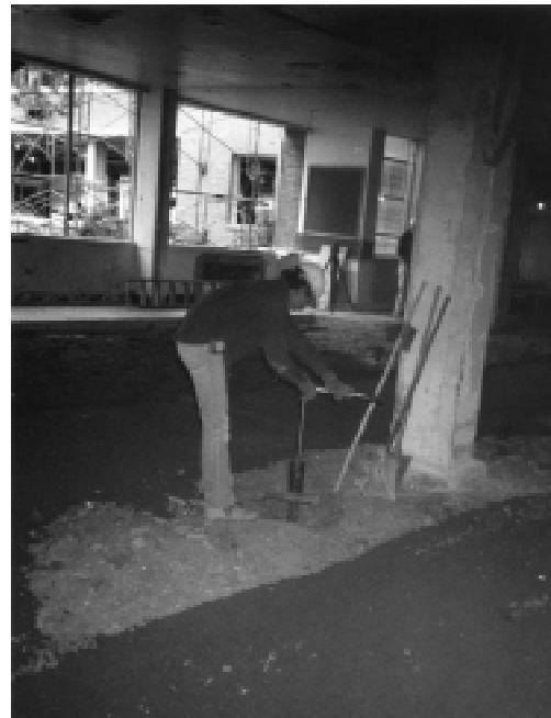
Fabricated cap with bolt allowed for precise adjustment with a laser level providing a reference point
