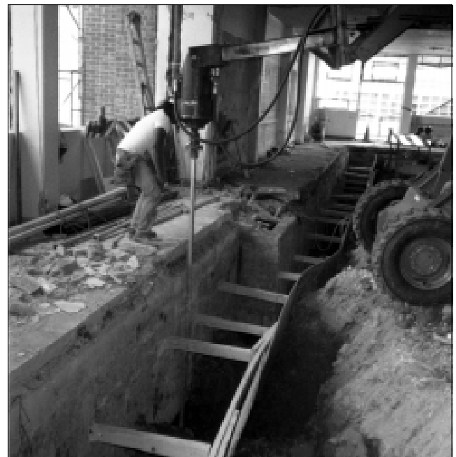
5,000 ft.-lb. hydraulic drive attached to skid loader installs screw anchor along side a utility vault
